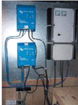
Turbine control unit and Inverters
